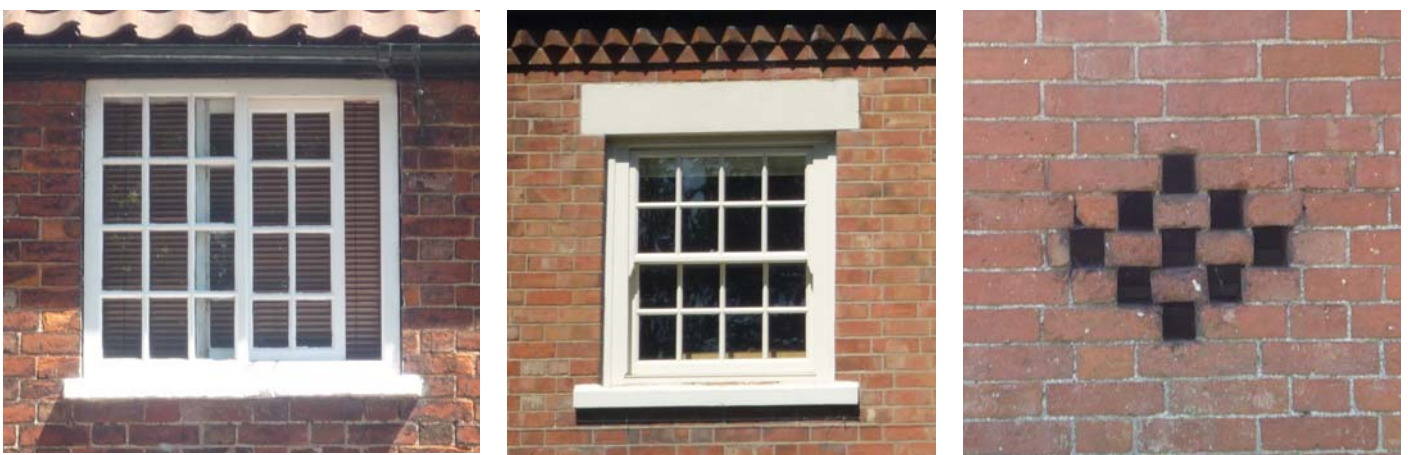
Above (left to right): Yorkshire (horizontally sliding) sash window; vertical sash window; missing brick ventilation patterning.
