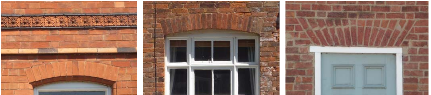
Above (left to right): flower patterned and jutting string courses; arched brick lintel; chamfered brick lintel.
