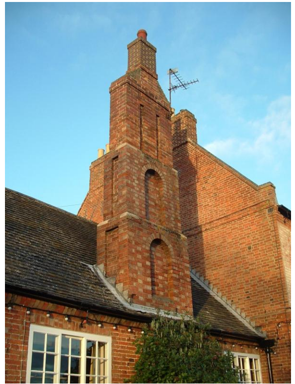
Three stage reducing chimney stack on the brew-house of the Unicorn's Head.
