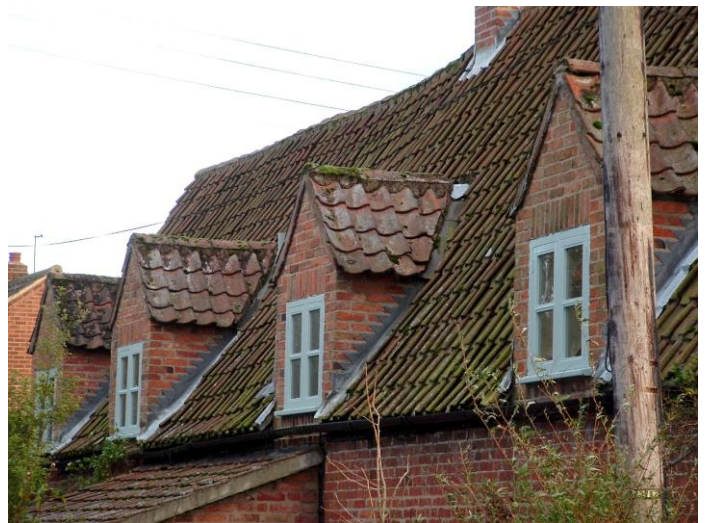
Orange clay pantile roof with timber casement dormer windows (Church Cottage). The steep roof pitch indicates that the building was originally thatched before the pantiles and dormers were added in the 19 th century.
