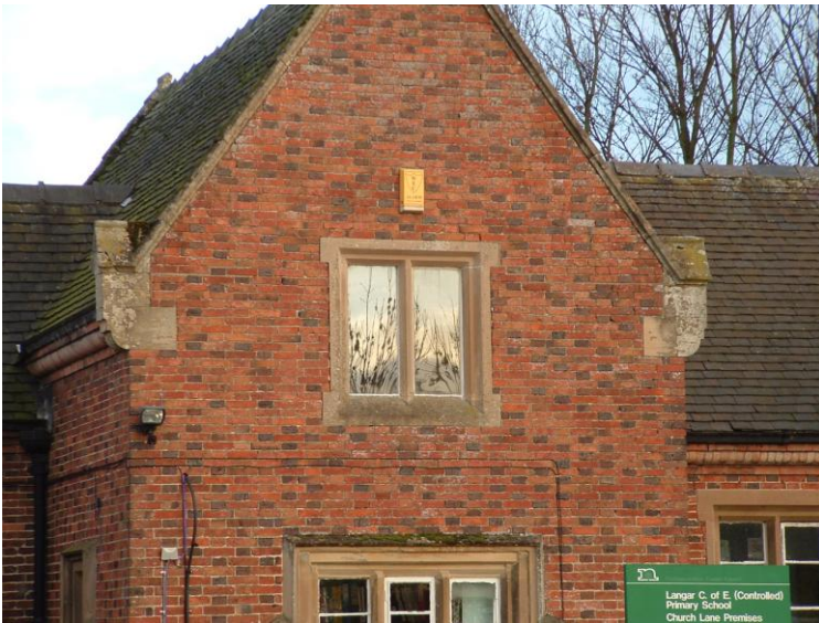
Ashlar mullioned casement window, ashlar gable copings and kneelers and blue brick headers (Langar Junior School).
