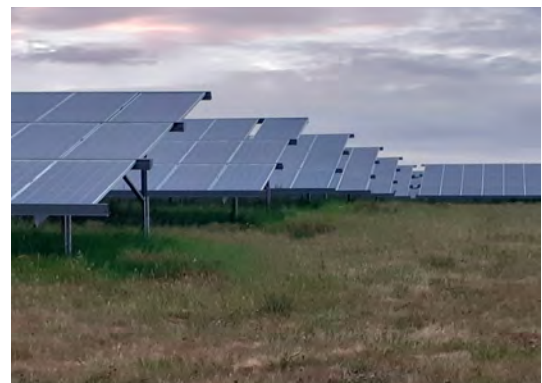
Solar Farm at Gedling Country Park
