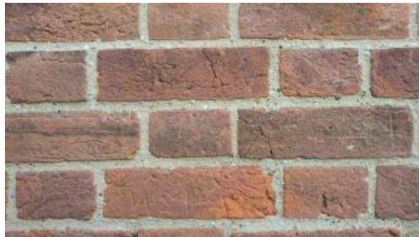
FIGURE 25: EXAMPLE OF NEAT MODERN POINTING, REGULAR JOINTS WITH THE EDGES OF THE BRICKS CLEARLY DEFINED
