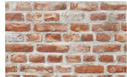
FIGURE 23: EXAMPLE OF POOR POINTING WITH WIDE JOINTS AND MORTAR SMEARED OVER THE FACE OF THE BRICKS
