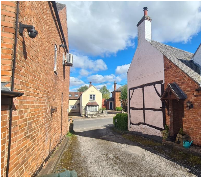
Figure 25 - Timber frame revealed on the side of a whitewashed house fronting Main Street (Zone 3)
