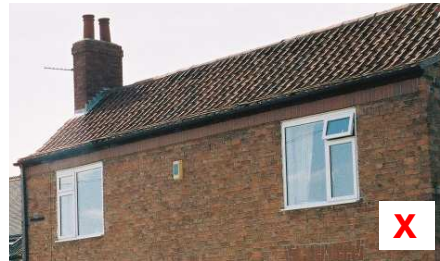
These modern windows are not in the style or materials of the originals and the window frames have been made flush with the facade – this single alteration has completely changed the character of this farmhouse.
