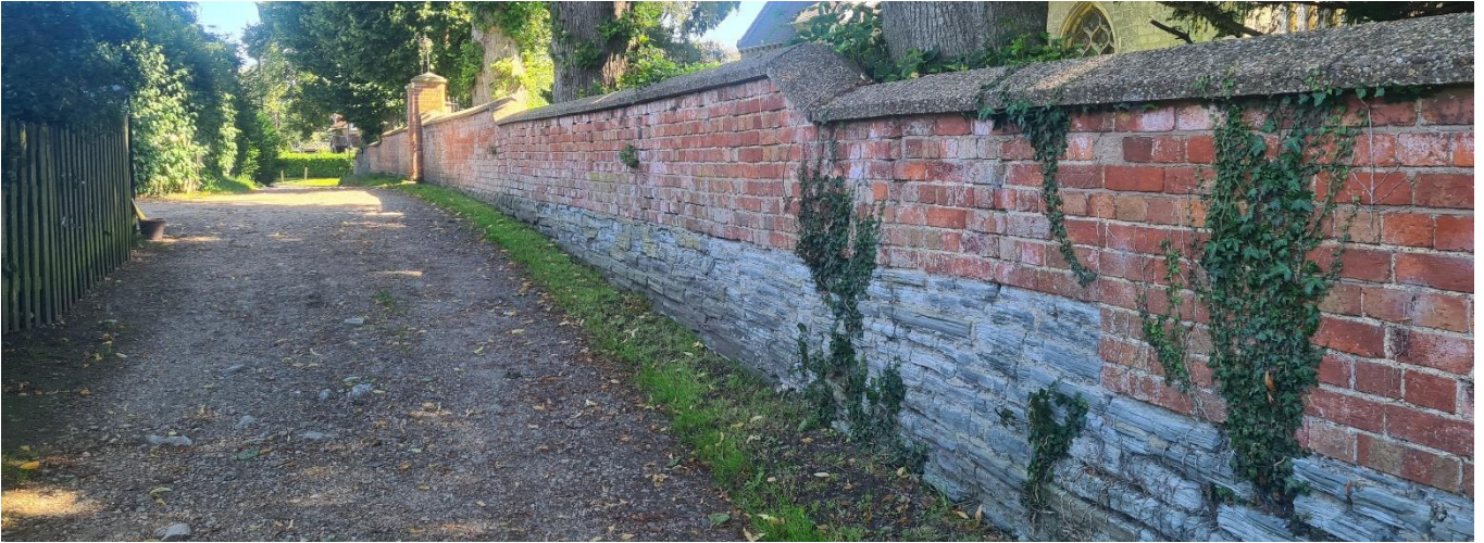
Figure 14 - Pathway and Wall Adjacent to St John of Beverly Church, Church Walk, (Zone 1)
