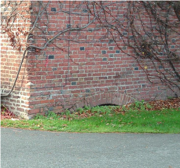
Brick wall with load bearing arch at foundation level, a common feature in Sir Thomas Parkyns' designs.
