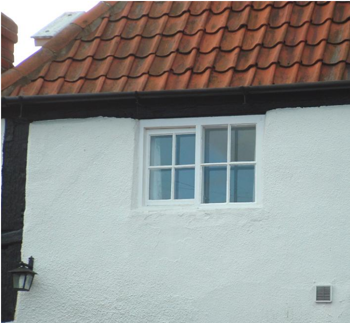
Timber Yorkshire sliding sash window, orange clay pantiles and whitewashed lime rendered wall.
